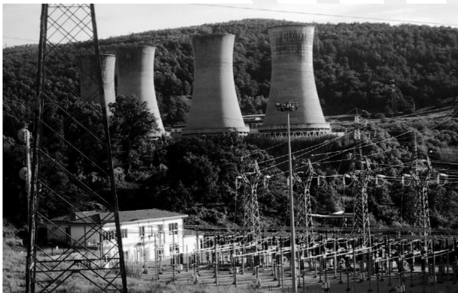
Fig. 7: Where world geothermal power production first started, Larderello, Italy. Site of the first experiment to use geothermal steam to produce electricity, on July 15, 1904, then site of the world's first geothermal power plant, 250 kW e , in 1914. Larderello, located on the hottest geothermal spot in all of Europe, today produces about 400 MW net of geothermal electric power.
